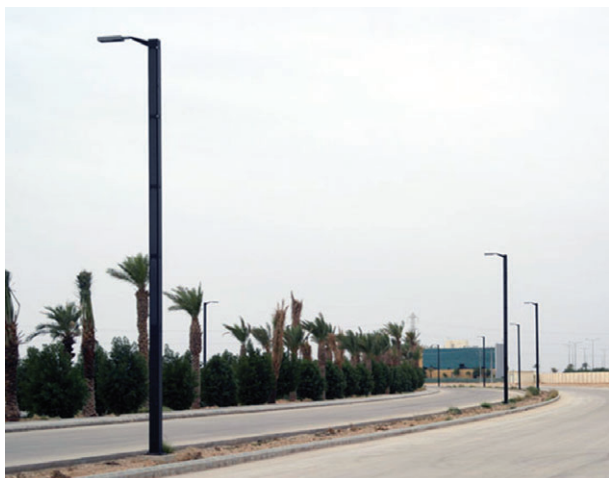
FIGURE 2 | Some of the 136 Monopole poles installed in Riyadh, Saudi Arabia. [Photo courtesy of Scotia, Vedbaek, Denmark].
