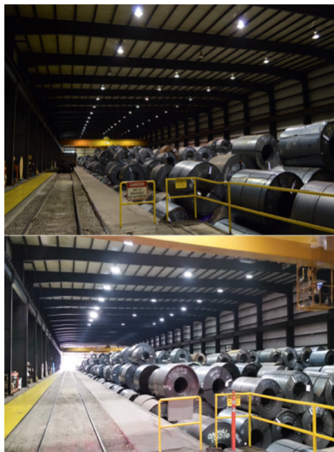
Fig. 2. The steel storage area at a US-based steelmaker lit with conventional fluorescent lights (top), and after retrofit with intelligent LED lights. Measured savings of energy for lighting across the whole company (Kenwal) go beyond 90%. (Image courtesy of Digital Lumens).
