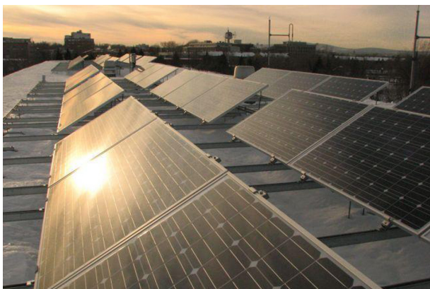
Figure 2. Since early 2012, the “Drolet” building of Quebec’s municipality hosts 60 PV monocrystalline silicon modules each of 250 W nominal power. (Reproduced from Ref. [14], with kind permission).
