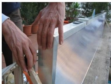
Figure 4. Installation of a glazed solar–thermal air collector on the balcony of a city building in Palermo, Italy.
