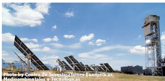
Fig. 14 In March 2008, a 100 kilowatt reactor for producing hydrogen through water splitting using solar energy was put into commission at the Plataforma Solar in Almería as part of the Hydrosol project. The reactor is located inside the tower on the right. (Reproduced from hydrosol-project.org, with permission).
