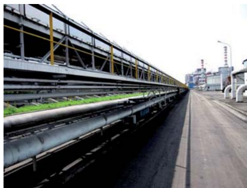
Fig. 2 First in the world to operate on such a scale, the 12 MW combined cycle plant in Venice's industrial zone of Porto Marghera fuelled by hydrogen by-products from local petrochemical industries. (Photo courtesy of Enel).
