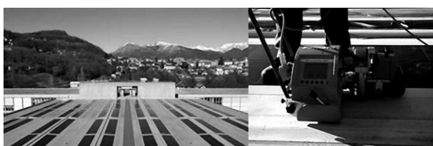
Figure 9. Thin-film PV modules laminated together with polyolefin membranes, which act as a waterproofing system. Roofing membranes are joined by means of hot air welding equipment normally used for the construction of flat roofs (reproduced from ref. [18], with permission).
